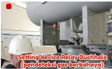
Setting piranti Relay Buchholz (Pendeteksi gas berbahaya)
