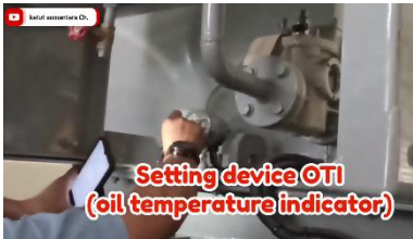
Setting piranti komponen OTI (Oil Temperature indicator)
